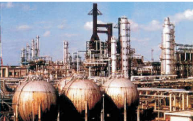
Oil Oil pumps, water injection pumps, compressors and so on
